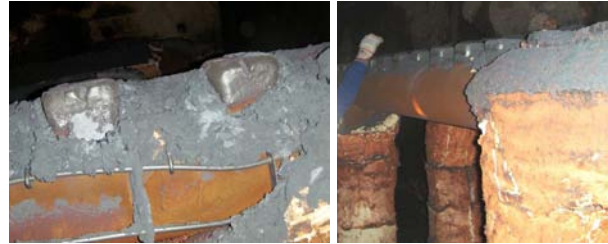
Fig. 1: Destroyed insulating modules made of RCF in WBF 1
