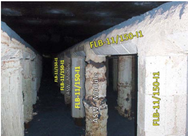
Fig. 6: Test area after installation of pre-fabricated shells made of light weight castable
