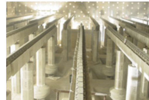
APPLICATION: Walking beam furnace
